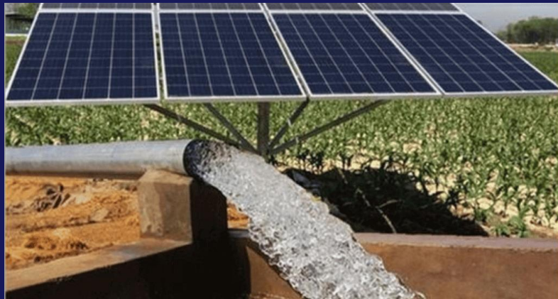
Solar Water Pumps
