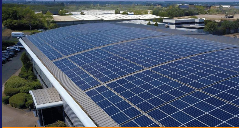
Solar Industrial Rooftop
