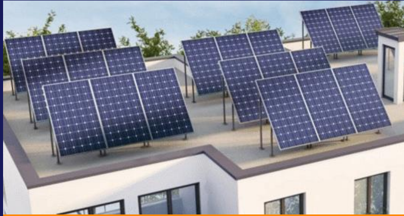
Solar Residential Rooftop
