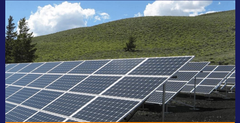
Solar Power Plant
