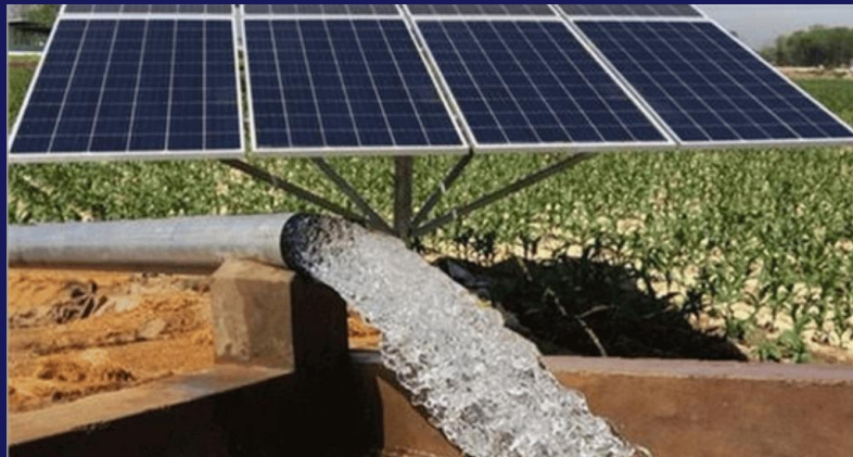
Solar Water Pumps
