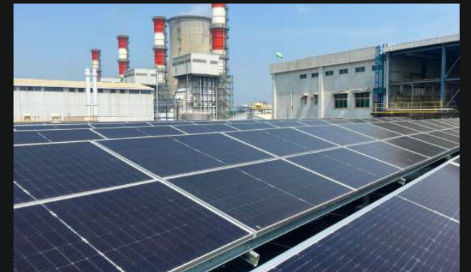
Torrent Power Surat, Gujarat 275 KW
