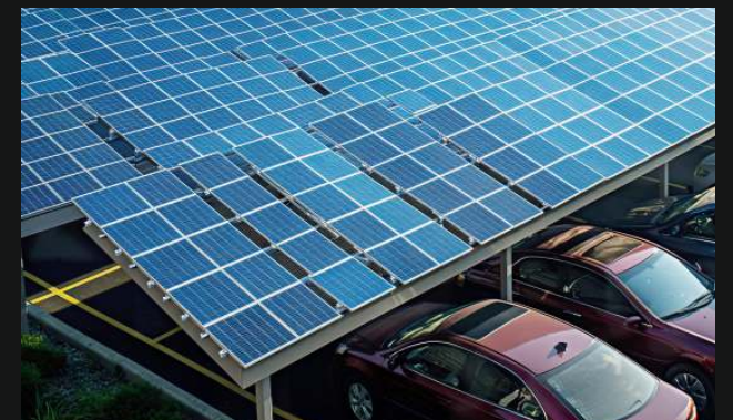
GoodLuck Textile Market Carport Surat, Gujarat 50 KW
