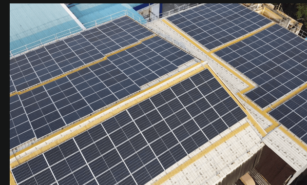
Agrawal Textile Mill Surat, Gujarat 260 KW
